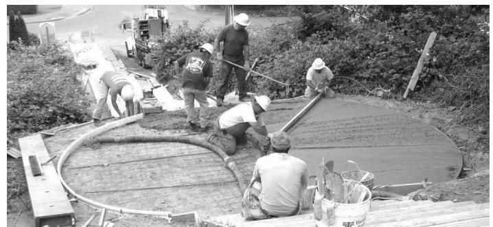
Seattle Dept. of Transportation crew pouring the Hillclimb stairway landing. After the landing was poured, they stamped a pattern of raindrops and cherry blossoms. Photographer: Judith Yarrow
